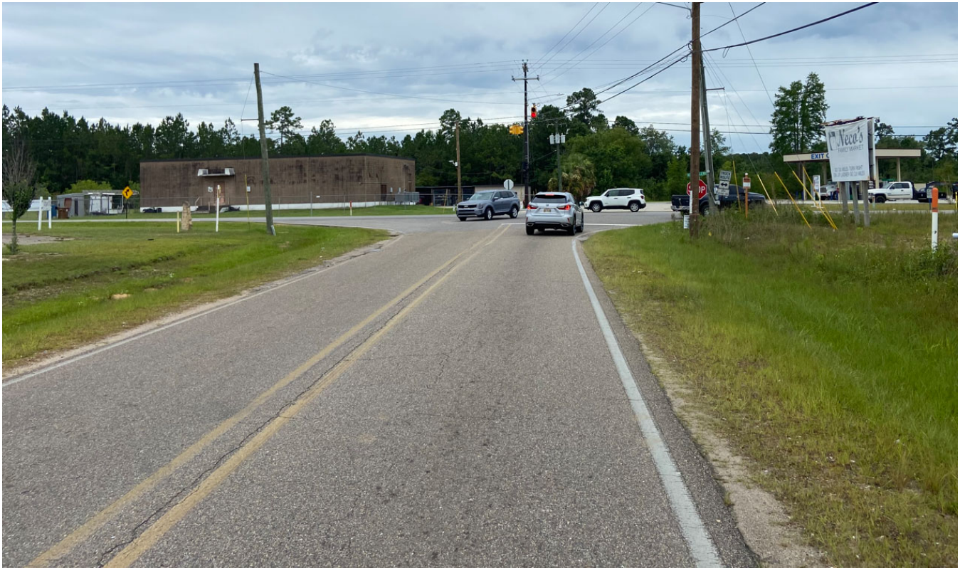
Above: Looking south on Edwin Ladner Road at Kiln Delisle Road with obscured Stop sign.
